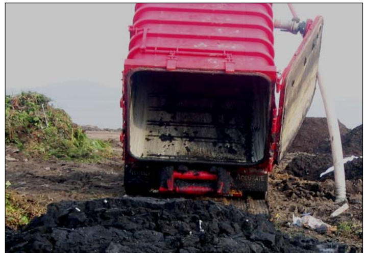
Job completed. Once the Oakland sewer main was cleaned, product collected by the patented closed-loop Sewer Hog™-Grit Gator "Paint Filter-dry" process was disposed in a landfill without further treatment.
