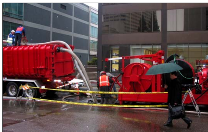
Jet setters. Workers in Oakland, Calif. are operating the Sewer Hog™, a patented, high-power water-jetting system specifically designed to clean out large-diameter sewers without taking the line out of operation and without releasing offensive odors to the surrounding area.
