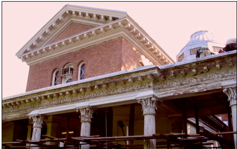
Paradise's craftsmen cleaned the façade carefully to avoid damaging the structure, using gentle water pressure and a minimum of chemical cleansers.
